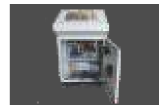
State of Art Electric Control Panel
